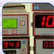
level control sensors
