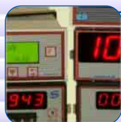
level control sensors
