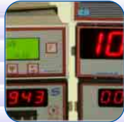
level control sensors
