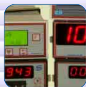
level control sensors
